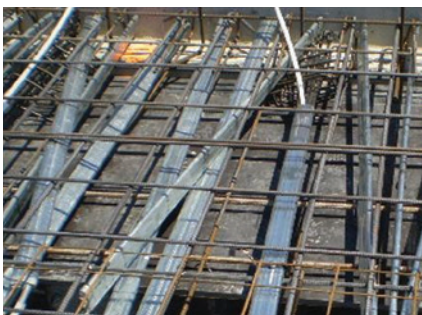
The performance of site assembled systems can be unreliable
