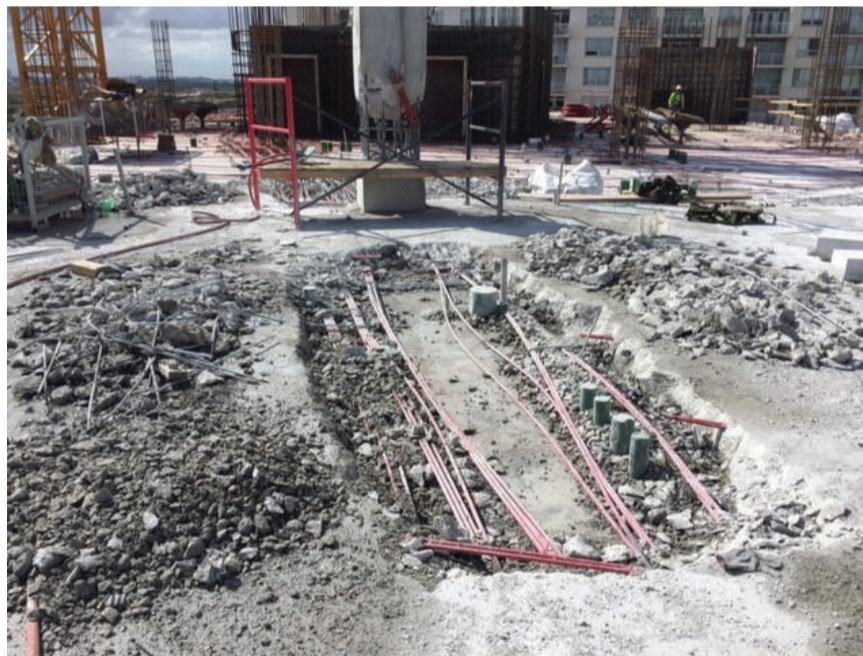
Figure 6-4: Example of damages due to early post tensioning
